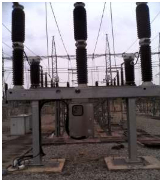
Figure 1: 132kV, PINGGAO GROUP Circuit breaker
